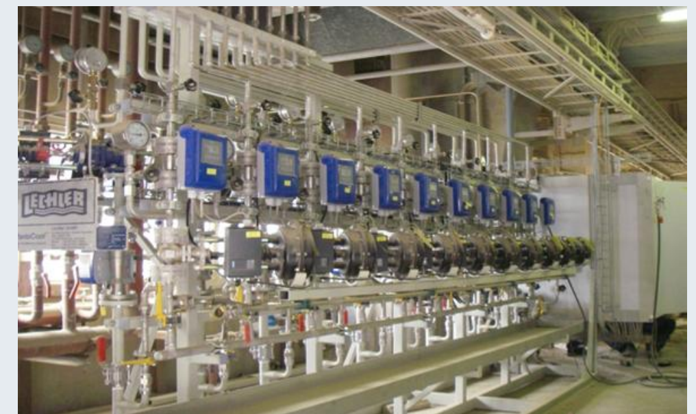
Control skid for of a high efficiency SNCR-system
